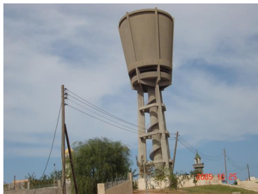
Figure 3: Photo of inactive elevated tank due to structure design faults in Central Tripoli Municipality [1]
