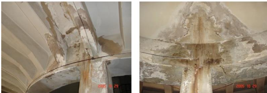
Figure 4: Photos of inactive elevated tank due to water leakage
