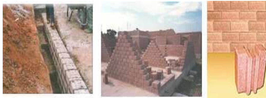
Figure 2: The bricks being laid with mortar, this is only necessary when laying the foundations, the rest of the wall is dry stacked [5].
