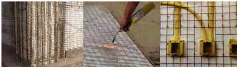
Figure 8: The propane torch trims back the polystyrene foam cleanly and neatly for installation of rebar, plumbing installations, and electrical conduit [6].
